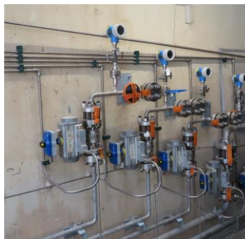
Figure 10 : Part of the new liquid fuel supply
