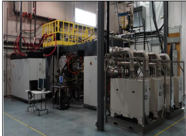
Fig 1. Tekna ICPT 350 kW Tunnel
